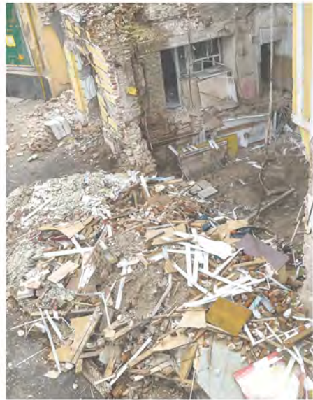
Photo of Pavlov Building rubble
